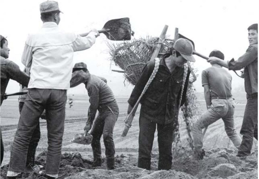
Village people participated in the embankment construction at Wangsuk stream in Namyangju
