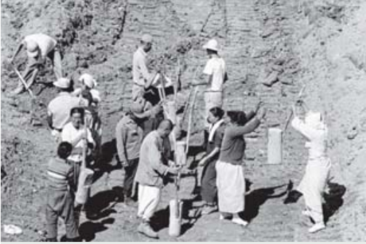
WFP's beneficiaries ramming down soil with wooden pounders for the construction of a water storage dam
