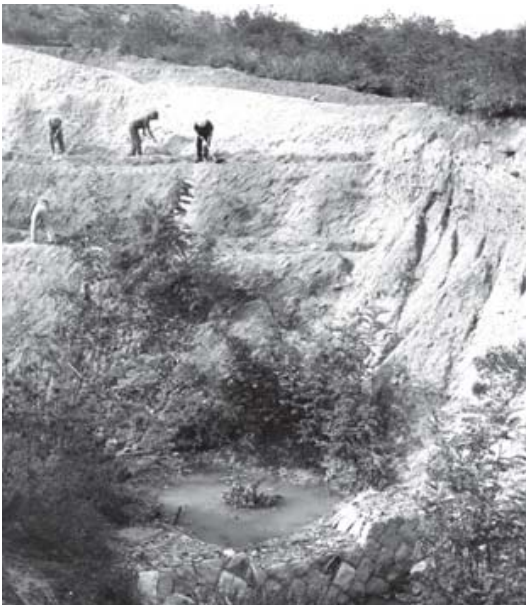
Landslide control work in progress in an area of sheet erosion and gully erosion
