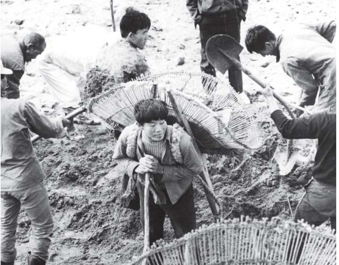
People working on the reinforcement of river banks along the Mushim stream in Cheongju district
