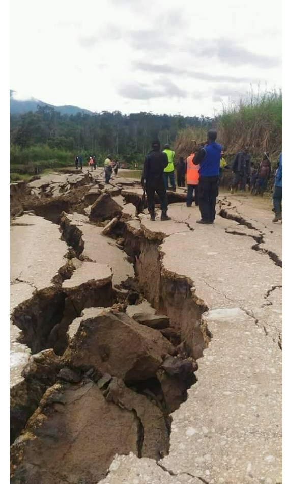
Moro Road damaged-Maggy
