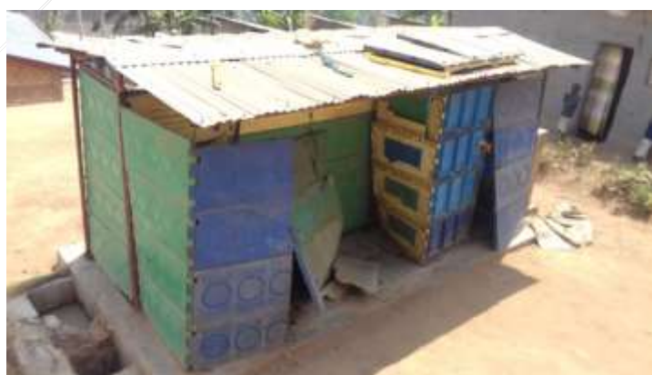
Figure 10: Older shower blocks in Mugombwa camp, August 2017
