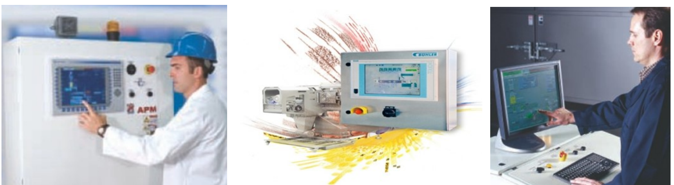
Figure 22: Extruder control units close to the extruder and as well in the control stand
