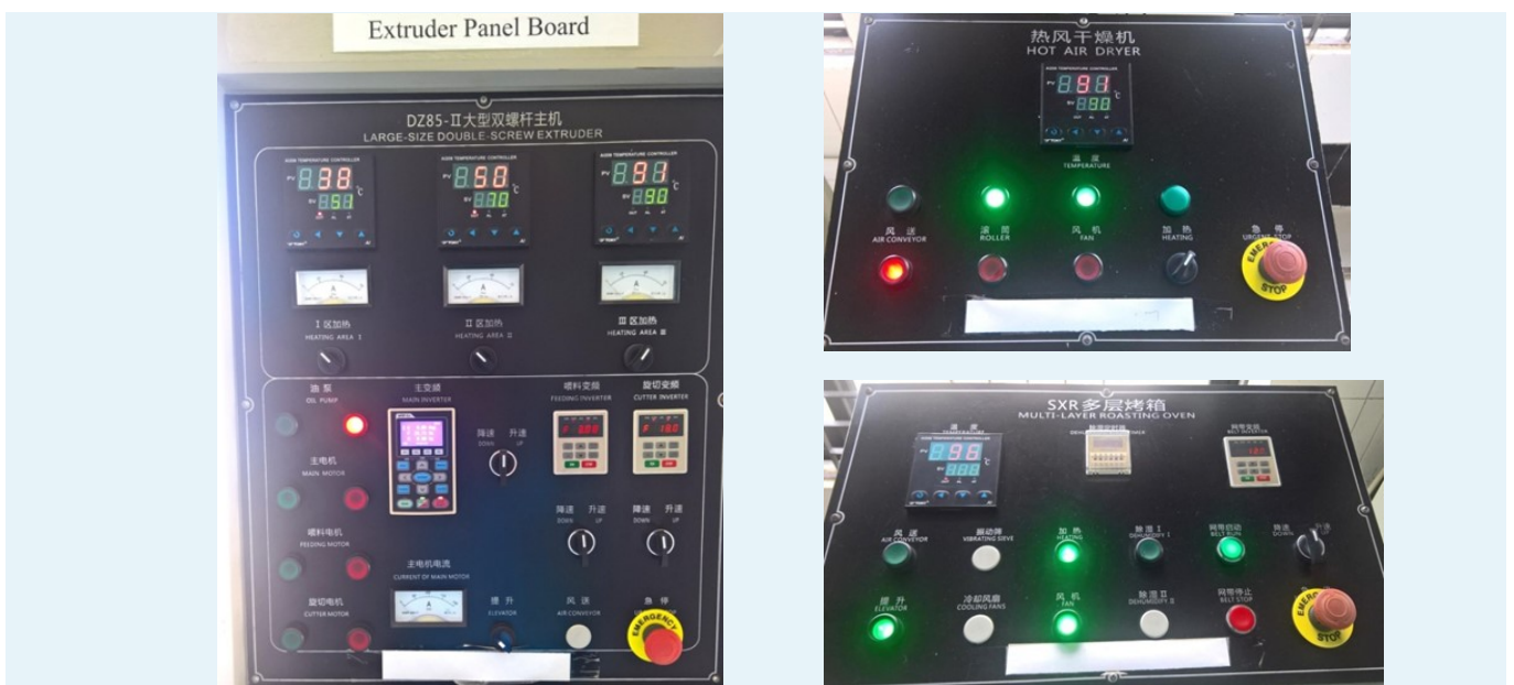
Figure 21: Control panels from a warm extrusion process installation
