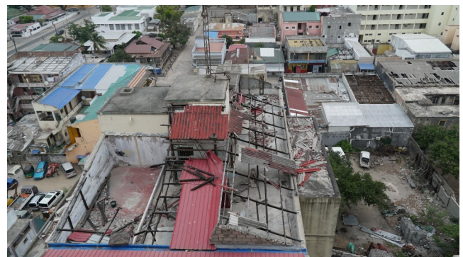
Hospital destroyed by TC Idai in Beira city, capital of Sofala province
