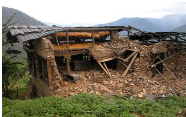
Caption: A house damaged by an Earthquake in Bhutan
