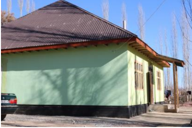
Photo: WFP supported the construction and rehabilitation of houses affected by earthquakes in Tajikobod District. ©WFP
