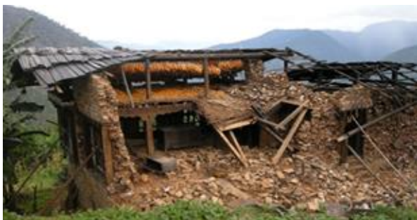
A house damaged by earthquake in Bhutan
