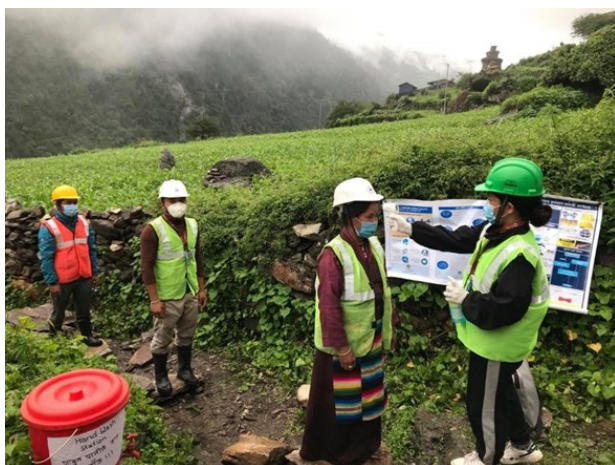
Photo 1: Health and Security Officer checking body temperature at construction site under Post Earthquake Recovery/ PURNIMA project, Photo by Suraj Kandel.
