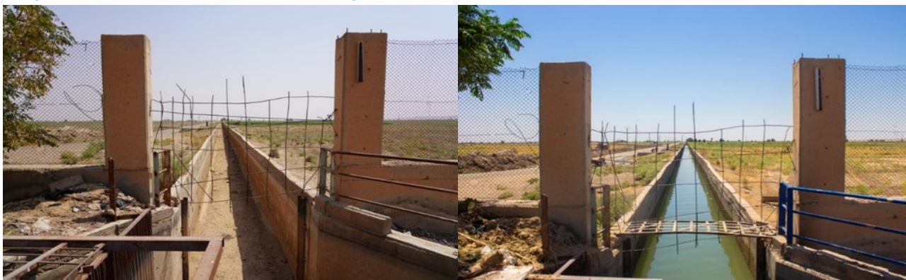
Figure 18: Water flow in Sector 5 main irrigation canal before and after rehabilitation in December 2020
