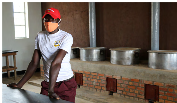
Through its Home-Grown School Feeding programme, WFP supported the construction of new water, sanitation and hygiene (WASH) facilities – including new fuel-efficient stoves – throughout schools in Rwanda during the COVID-19 pandemic, in partnership with World Vision International. © WFP/Daniel Kibsgaard
