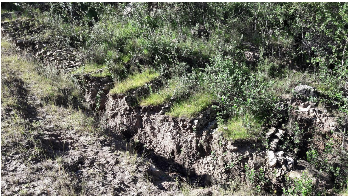
Photo 8: Collapsed check-dams due to run-off from a diversion furrow in Botha-Buthe
