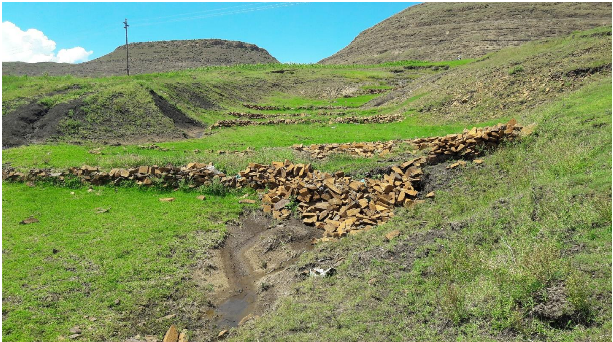
Photo 4: Collapsed check-dam without spill-way Ha Maneo Mohale's Hoek
