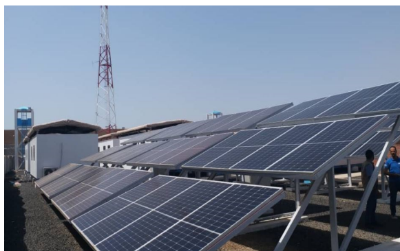
Solar panels in Mokha hub, Yemen.
