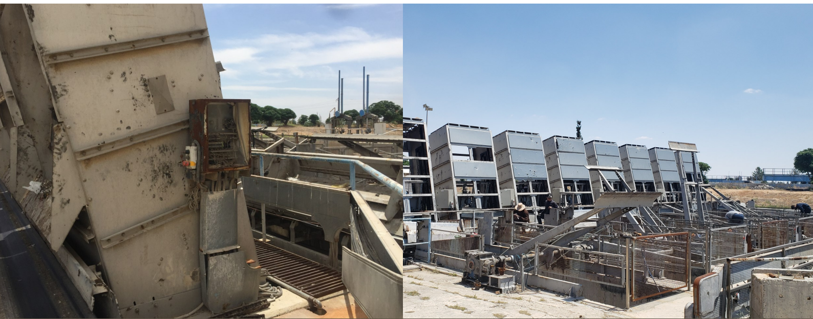
Before and after pictures of the plant rehabilitation. Photo: WFP/Country Office Engineering team
