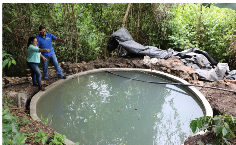
Rainwater collection system. Photo: WFP/Nicaragua Country Office
