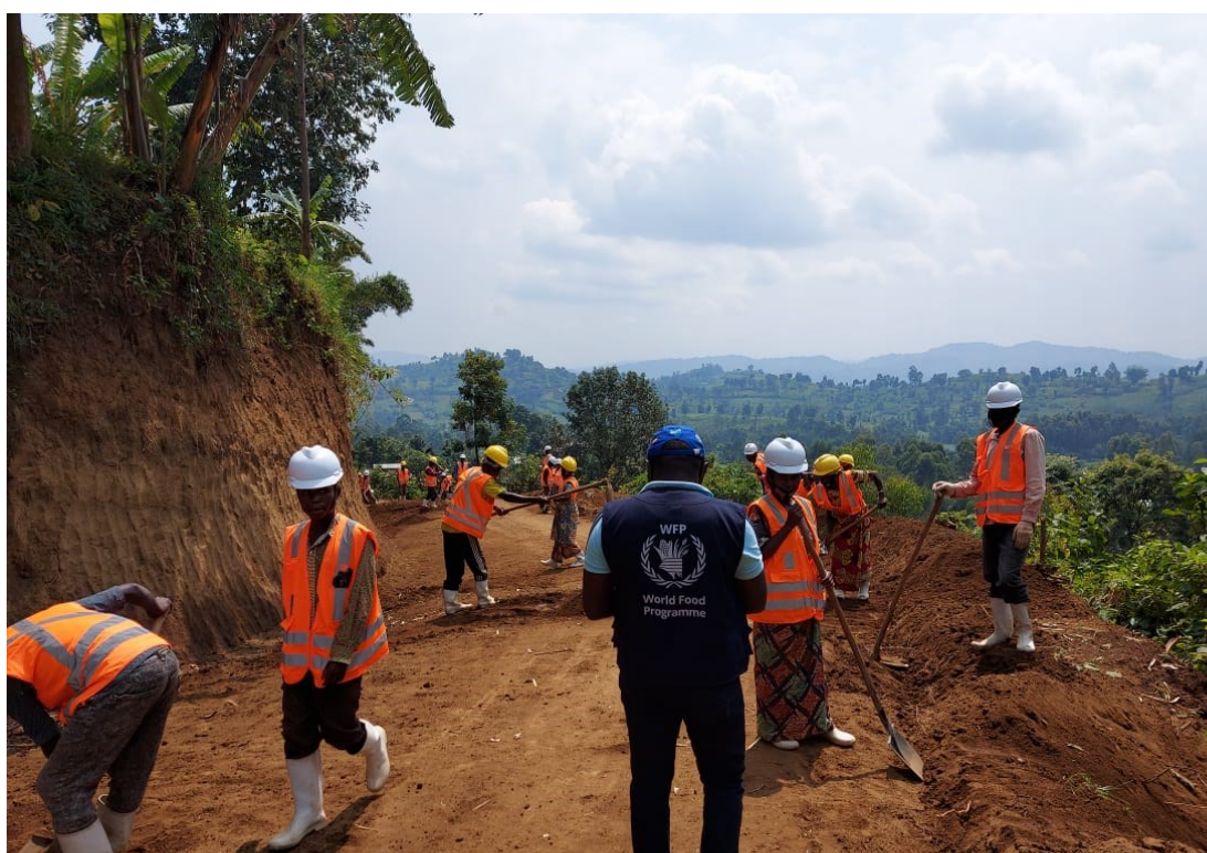
Community members carrying out road rehabilitation works in North Kivu. Photo: WFP/DRC Engineering team
