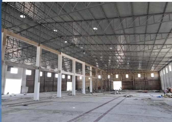
Construction process of new warehouse in Jijiga. Photo: WFP/Country Office Engineering team
