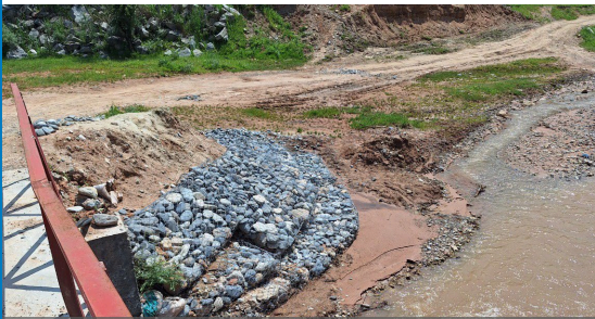
Riverbanks were reinforced with gabion nets as part of WFP's asset creation project to protect the village from floods, Bulolu village, Osh Province © WFP/Photo Library
