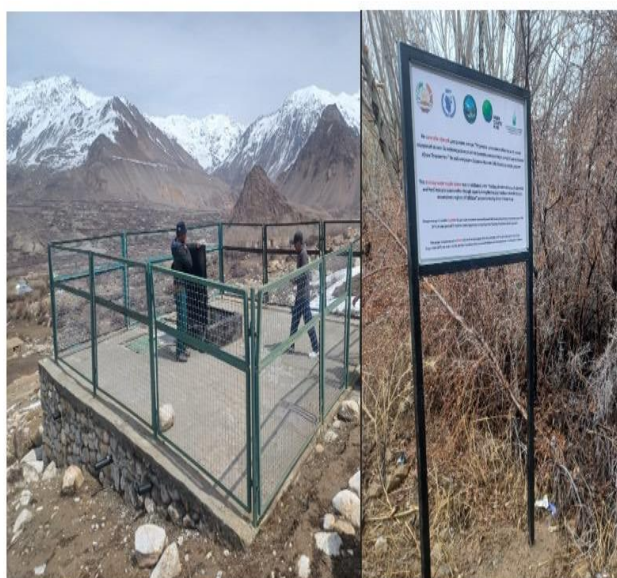
Drinking water supply system, GBAO Photo by Gufronjon Ayubjonov
