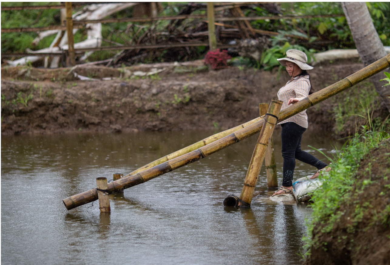
Community members from Davao de Oro worked on building a farm reservoir through the Government's Project LAWA, to mitigate the impacts of El Niño in 2024. © WFP/Earvin Perias
